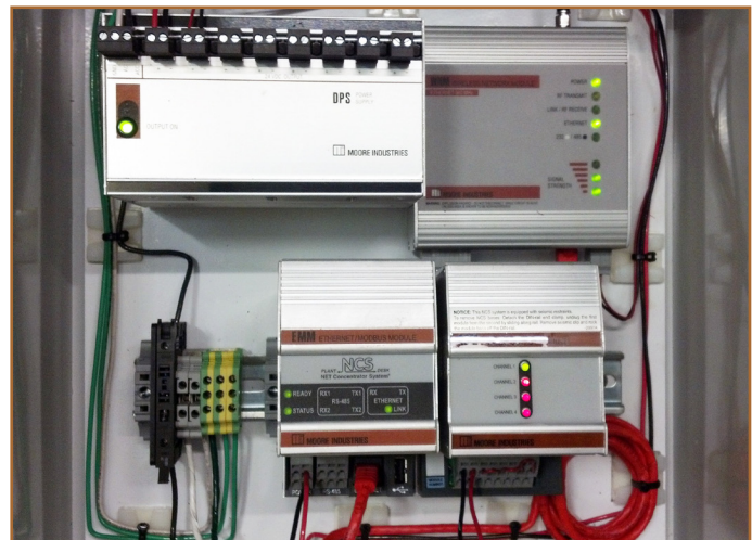
Figure 4. The wireless receiving panel installed at the boiler room of the pulp and paper mill. An EMM Ethernet/MODBUS Interface Module of the NCS NET Concentrator System served as a MODBUS Master to retrieve HART data from the HCS at the pond site.
