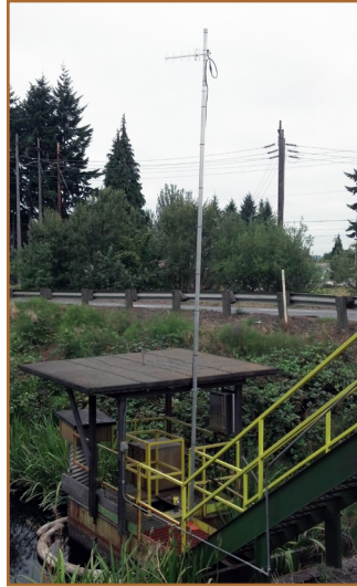
Figure 3. The Yagi-directional antenna was used at the pond site to transmit level signals from the HART level transmitter to the boiler room.
